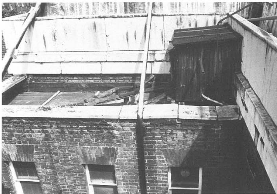
A detail of the dilapidated brick- and stonework. See page 51.
