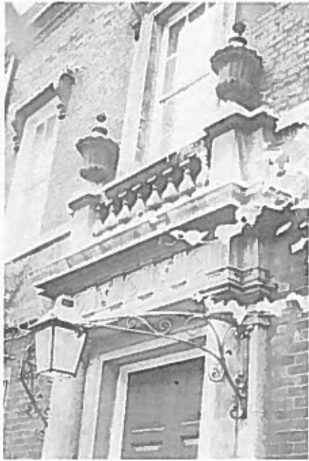
The King's Road palazzo. The doorway of Argyll House (left), designed by the Venetian architect Giacomo Leoni, who was also responsible for Moor Park in Middlesex and Clondon Park in Surrey. The house — 211 King's Road — was built in 1723. (See pages 43-4).
